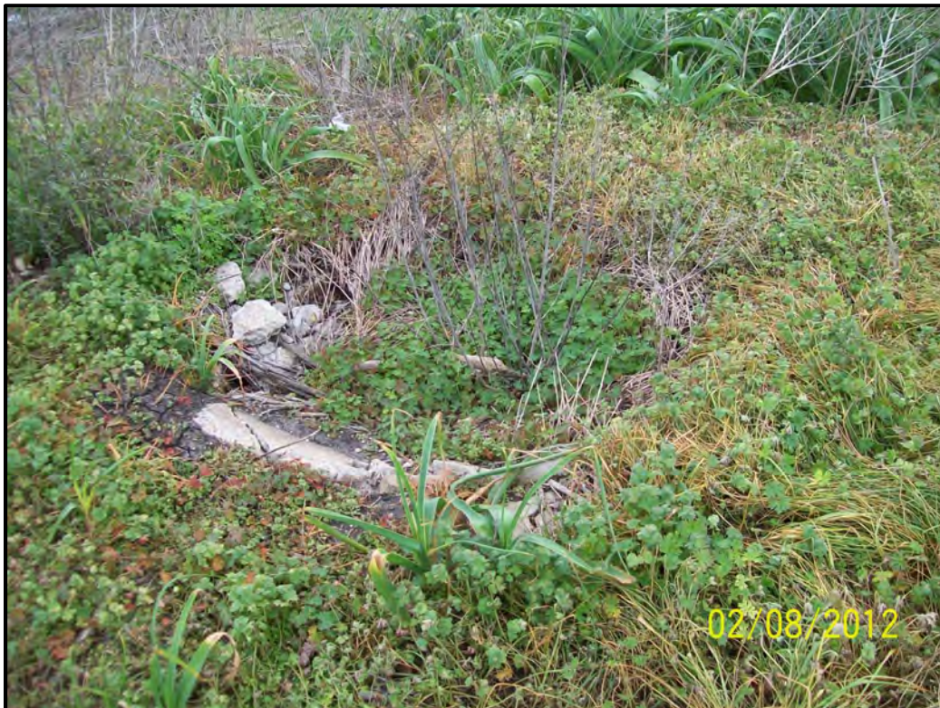
Photograph 14 – View of the filled in septic tank located adjacent to the water well and storage building.
