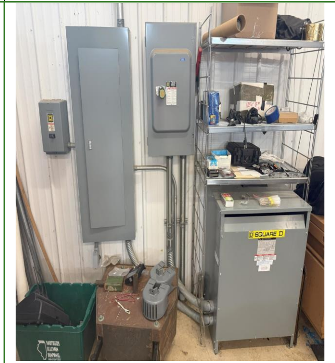
View of electrical panel and associated utilities in shop area
